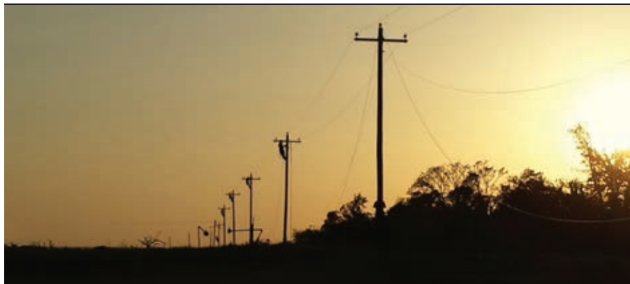
Look closely at the top of each pole to see crews putting the finishing touches on almost a mile of tornado-damaged line—rebuilt in a single day!
